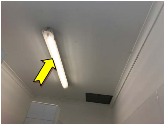
Photo 3. Interior, throughout, single tube fluorescent light fitting – suspected PCB-containing capacitors.
